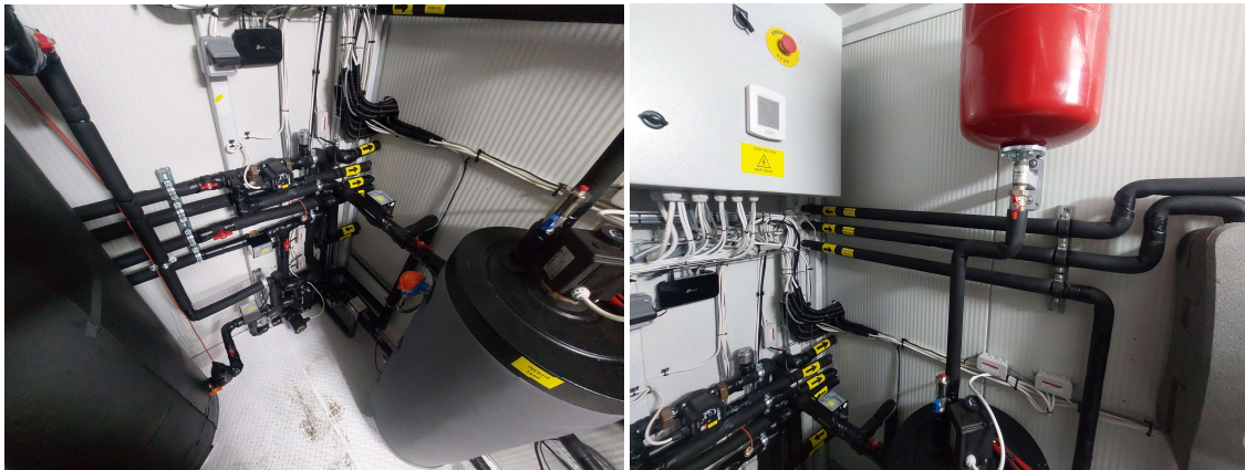
Figure 15. Water pumps and piping connecting the TCM with the solar inertia tank and the heat pump side.
