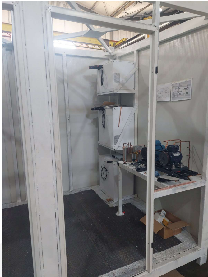
Figure 20. The PCM vessels and the heat pump circuit during manufacturing.
