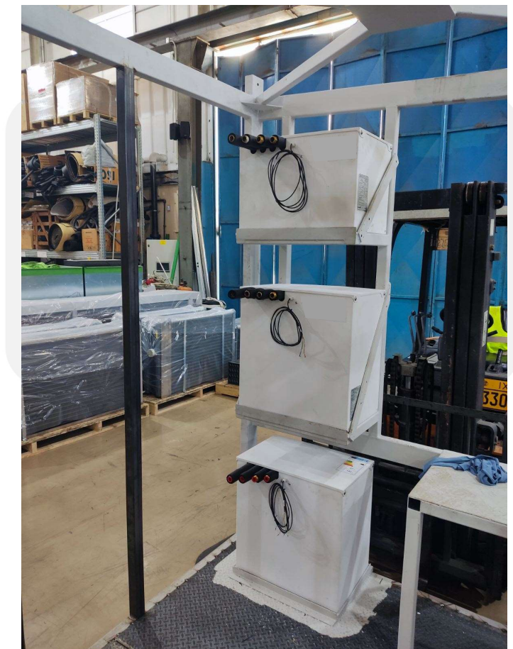
Figure 19. Placement of the PCM vessels on the metal frame of the container for all demo sites except Cork.
