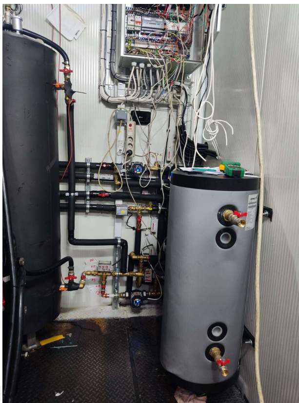
Figure 11. Coupling of the NH 3 circuit with the solar buffer tank and the electrical panel under manufacturing.
