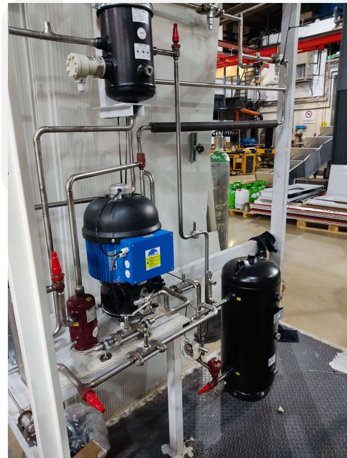
Figure 8. The NH 3 compressor, receiver and separator during the MiniStor assembly.
