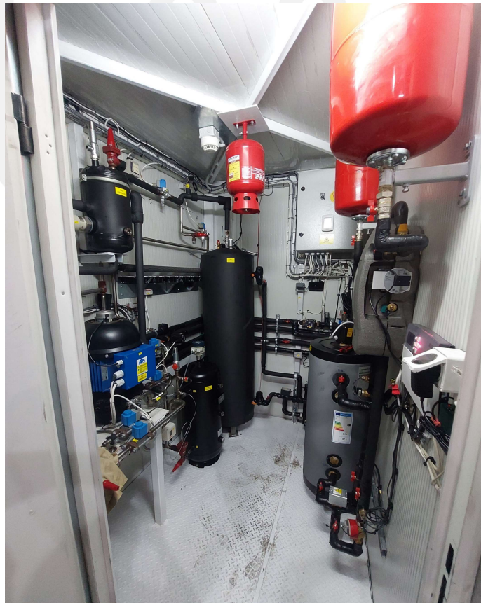
Figure 14. The TCM reactor integrated with the solar buffer tank circuit.
