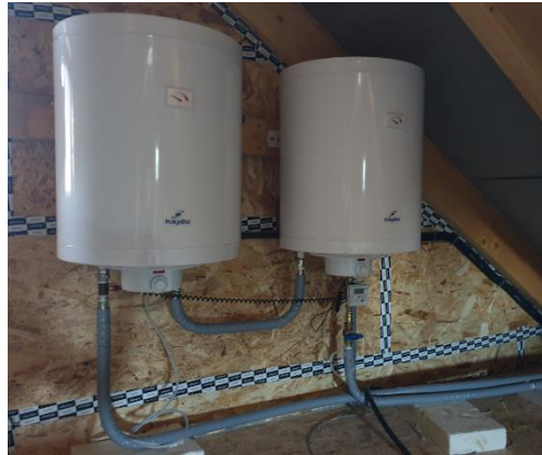
Figure 17: The two boilers providing DHW in Sopron demo site
