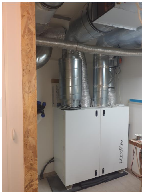
Figure 14: Central unit of airing system of Sopron Demo Site
