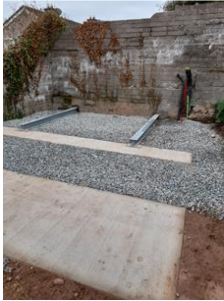
Figure 30: Installed foundations for the MiniStor container and the solar panel frame (Cork demo site)
