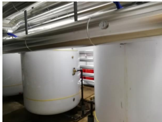
Figure 10: BC boiler room. Inertia Tanks (USC demo site).
