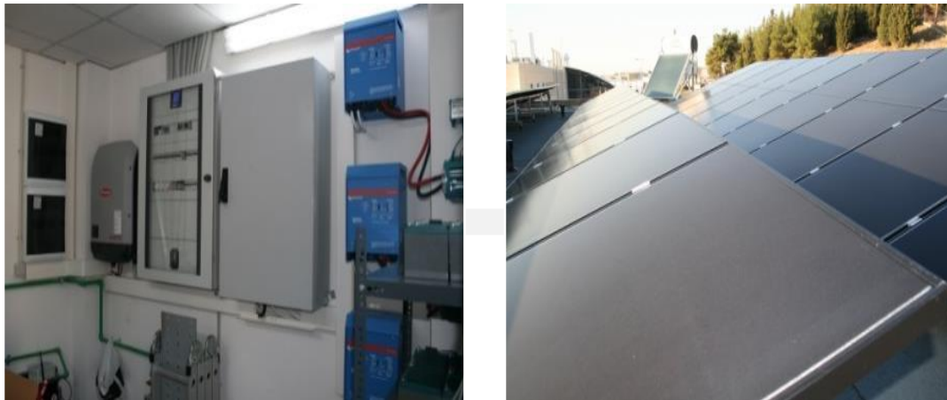
Figure 4. View of existing Smart Home's machinery room (left) and currently rooftop installed PVs (right).
